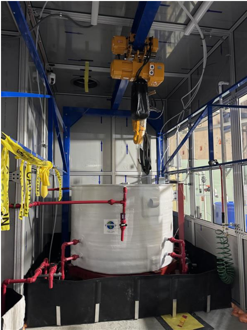
Walkdown of Blue Monorail Hoist
